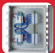
9. DC surge protection
